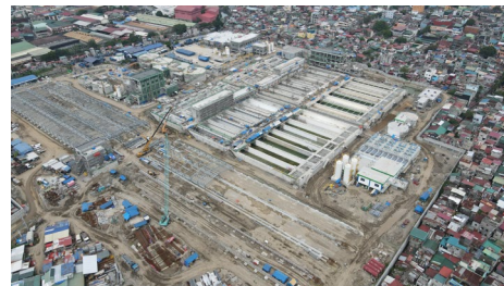
Camana Wastewater Treatment Plant
